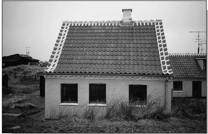
Figure 15.7: In exposed coastal areas of Denmark, the roof tiles along the ridge and the gables are fixed with lime cement mortar to prevent them blowing off.
